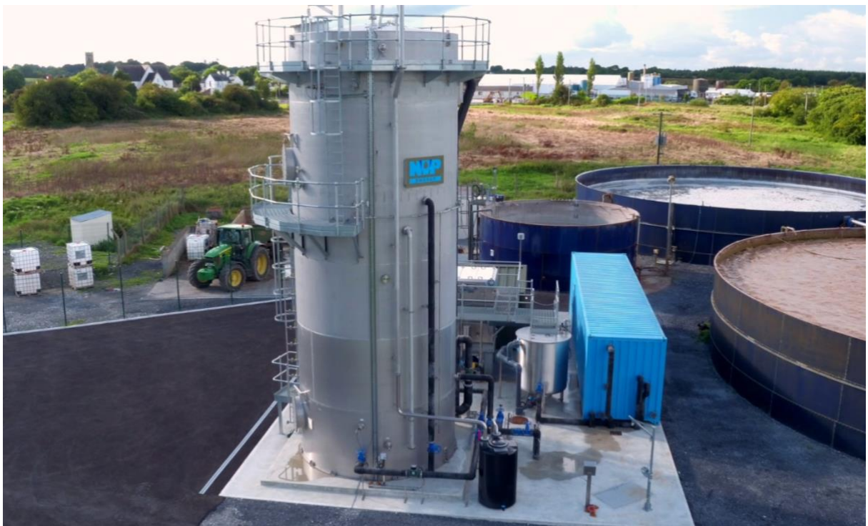
Figure 1: NVP Energy Anaerobic Treatment Plant at Arrabawn Co-op, Kilconnell, Co. Galway
