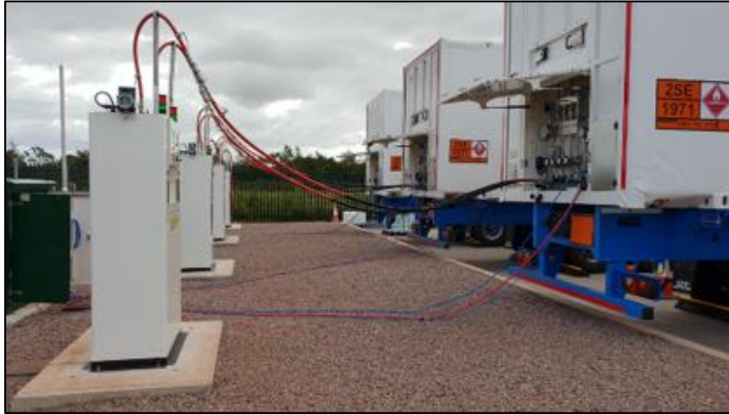
Trailers connected to dispensers
