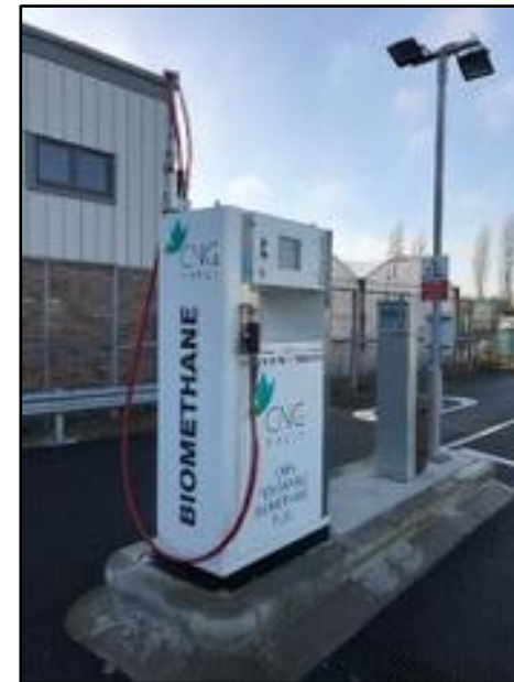
Dispenser & Fuel Management System (Leyland)
