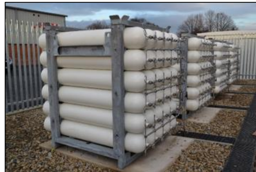
300barg CNG Storage (Leyland)
