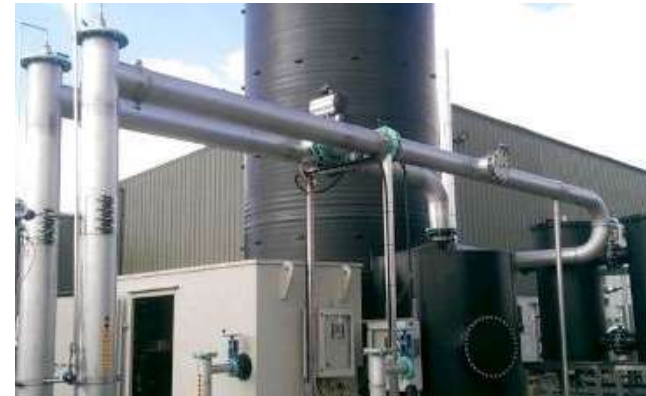
Figure: CSO scrubbing system
