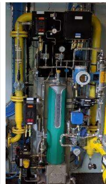
Propane mixing unit
