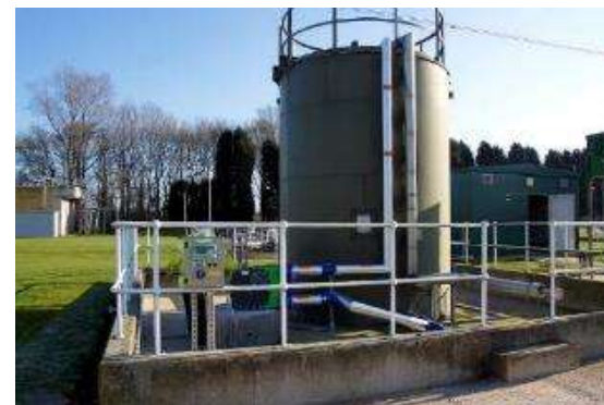
Figure: Example dosing tank and dosing pump arrangement
