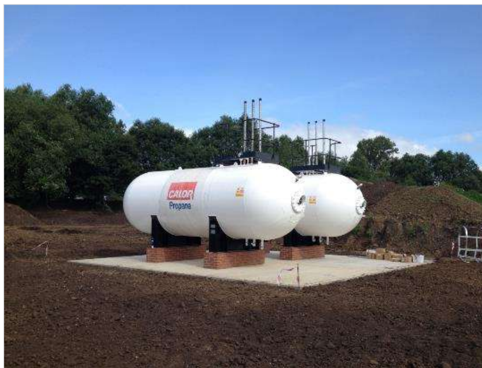
Propane storage tanks
