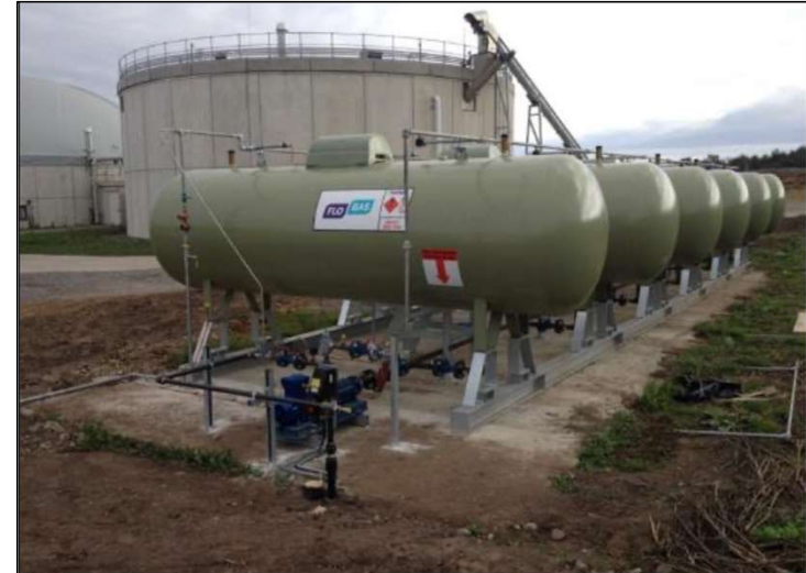
Above-Ground Propane Storage cng services 6 x 2 tonne tanks
