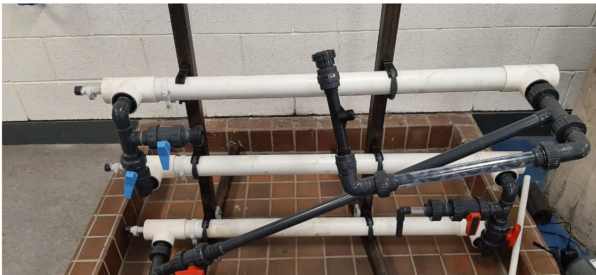
Fig. 3: “Triple-leg” system with in-pipe electrodes. We connected a raw-biogas cylinder to the upstream Venturi-system to allow for microbubble generation of the raw biogas, and subsequent in-pipe CO 2 capture.
