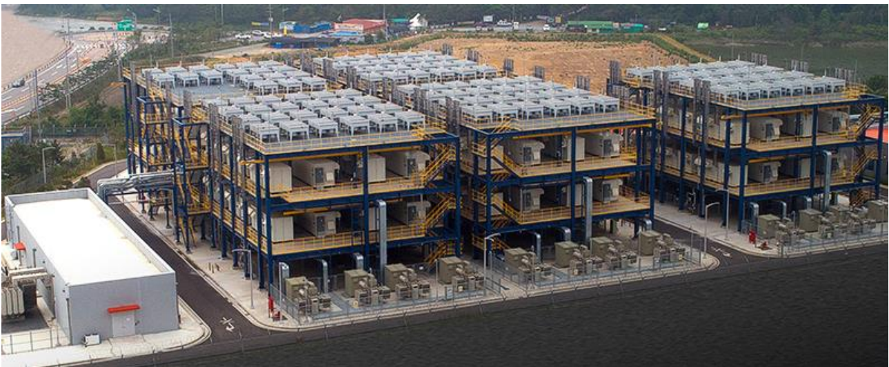
Figure 1: Fuel Cell Power Plant in Daesan Korea
