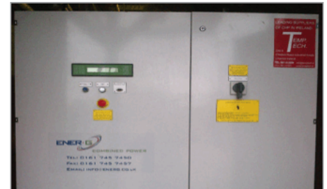
Figure 2. ENER-G Combined Heat and Power Unit
