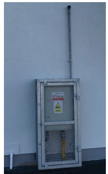
Natural gas meter with meter protection
