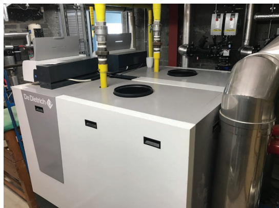
Natural gas boiler
