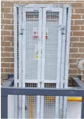
Figure 17: G160 MP skid unit with protection
