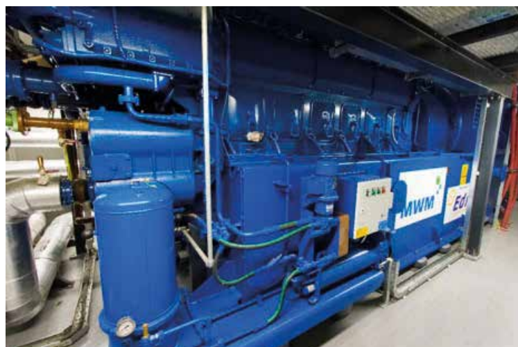
Figure 2: CHP unit in Bausch + Lomb factory Waterford
