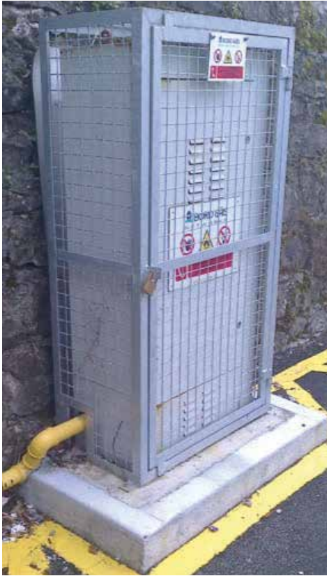
Figure 21: G65 MP module with protection (provided by builder)
