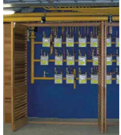
Figure 23: G4 meters serving retail units
