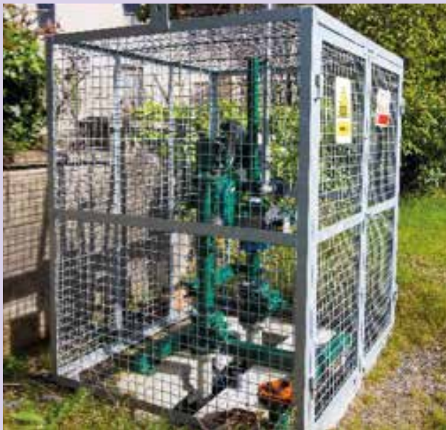
Figure 14: G100 meter with protection
