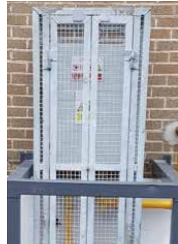
Figure 12: A G25 meter module with protection
