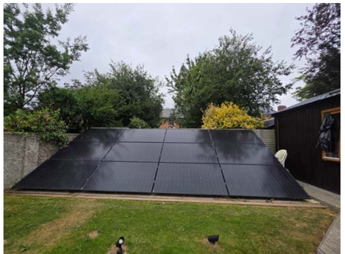
Picture 5: Finished 12-panel solar array with a 5.1 kWpeak output
