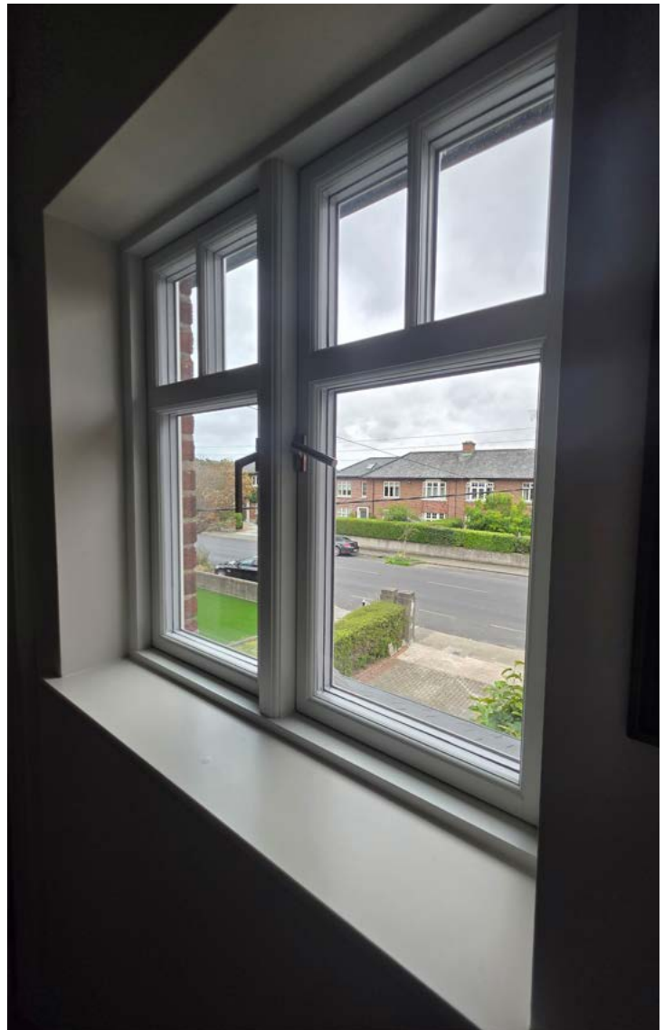
Picture 3: The modern triple glazed windows mimic the original windows from an architectural viewpoint while achieving the GreenFits Design Team requirements of airtightness and a U-Value of 0.73 W/m 2 .K
