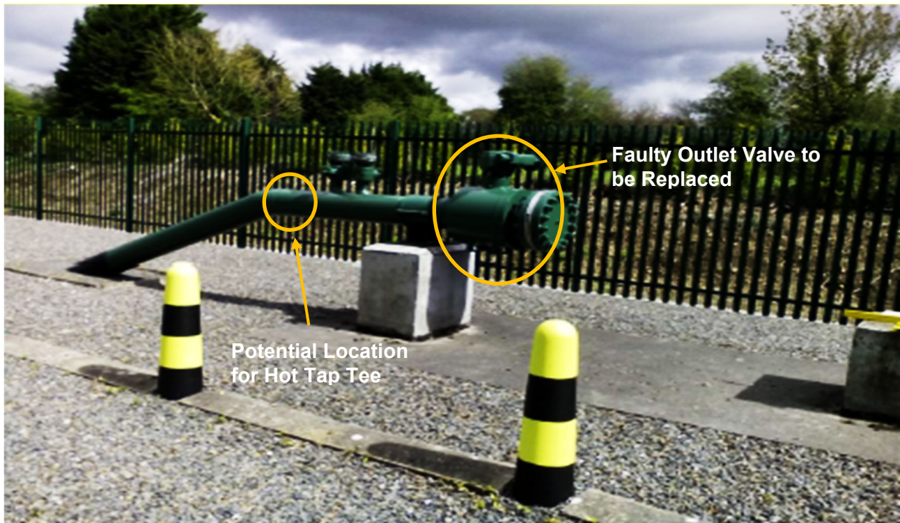
Figure 2-2: Ballynaclose Faulty Valve.
