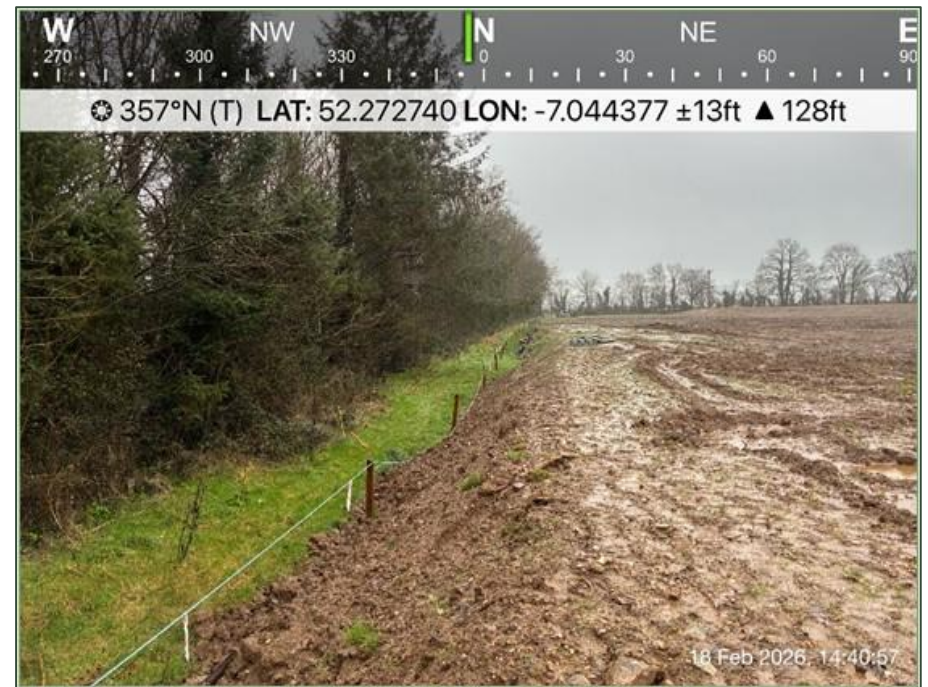
A2: View of the greenfield site currently under construction within which the pipeline will be installed.
