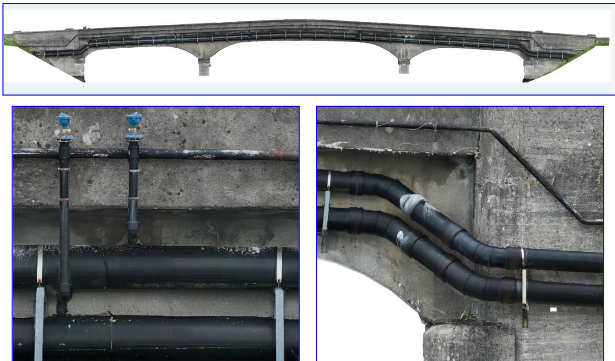
Figure 7 UAV close-range imagery of Ardnacrusha bridge gas pipeline crossing, Co. Clare, side-view orthomosaic (top) with detail views of pipe supports and fittings at bridge piers (bottom). Source: SurveyLabs Ireland [54]
