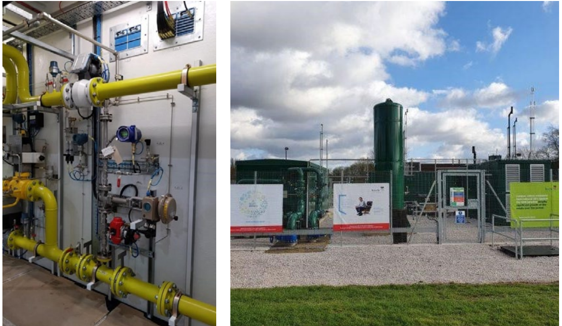
Figure 8.1 HyDeploy injection facility
