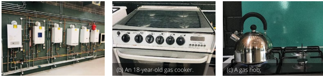
Figure 3. Appliances; (a) six condensing boilers, (b) an 18-year-old gas cooker, (c) a gas hob.
