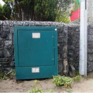
District Regulating Installation (DRI)
