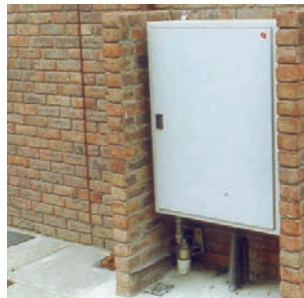
Six meter cabinet
