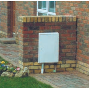
Domestic meter box
